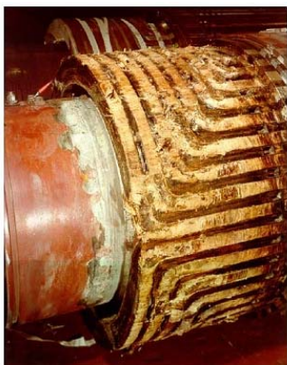
Turn insulation damage under retaining ring
